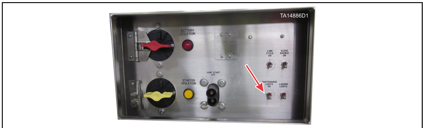
Figure 41: Maintenance lights switch
