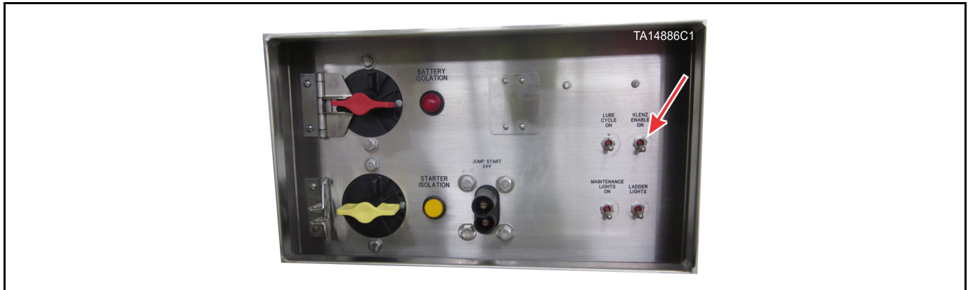
Figure 39: KLENZ enable switch
